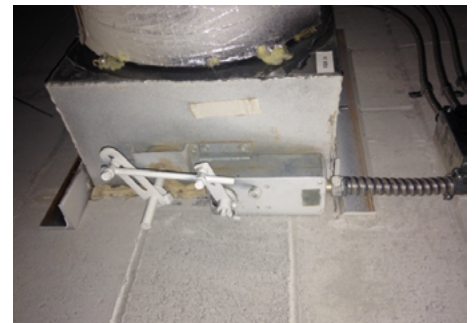
Figure 12.25 Linkaged motor here is typical of many applications.
