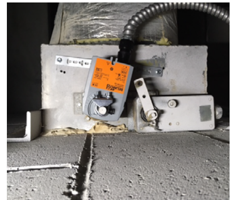
Figure 12.26 Belimo Replacement, the old motor remains disconnected.
