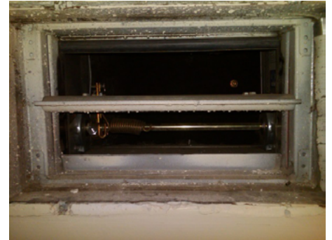
Figure 6.4: View of damper frame, blade, and shaft
