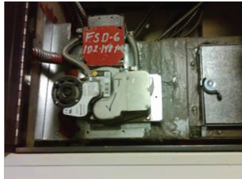
Figure 16.2: Externally mounted auxiliary switches
