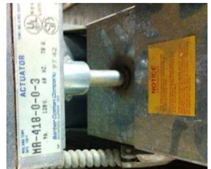
Figure 10.43 Detail of external coupling between motor and damper jackshaft
