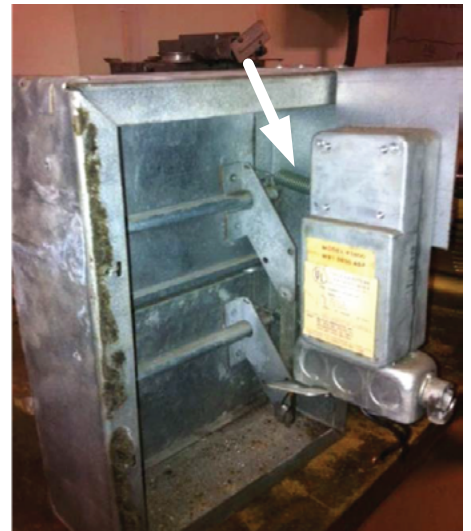
Figure 9.29: View from motor side
