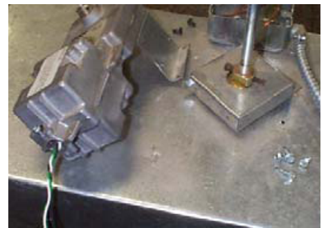
Figure 10.3: The old motor and spring are disassembled and removed. Then a Belimo can be direct coupled in the old motor's place.
