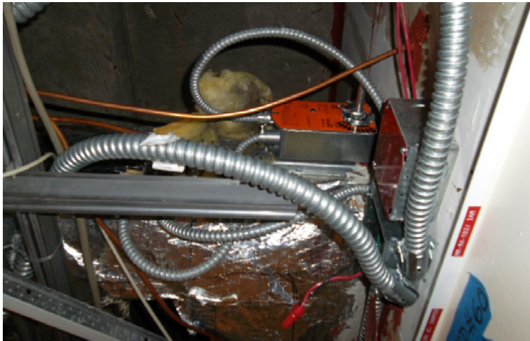
Figure 11.14 FSLF mounted in place of pneumatic actuator.
