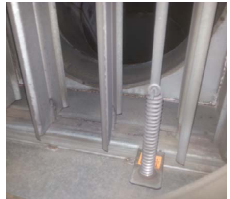
Figure 3.1 Typical existing installations
